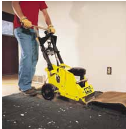
Quickly cut carpet in manageable strips for removal. With its large 8" tires, minimum effort is needed to propel the SFCS16.
